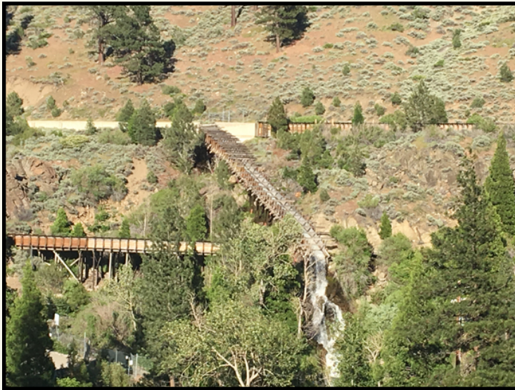
(Above) Spillway off the flume. Photo Courtesy of Kristen Sproat Colley, June 4, 2018.
