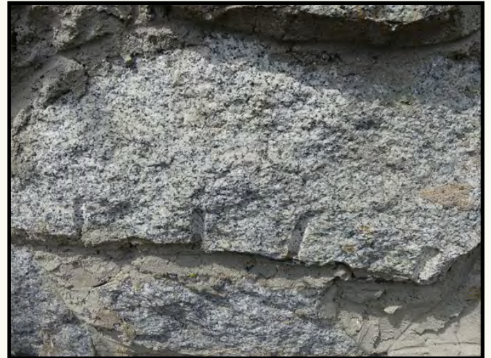
(Above) More evidence at McGlashan retaining wall
